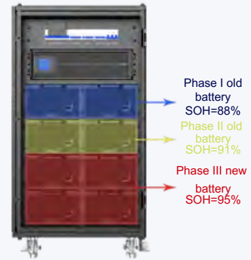
Mixed use with the old and new batteries
